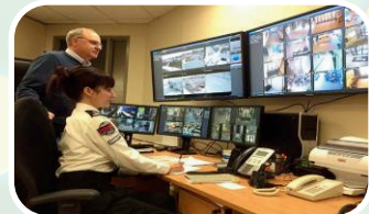
SECURITY AND SAFETY CONTROL
